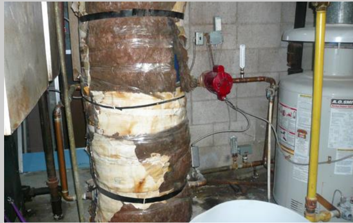
BOILER – 700 Ross St., Burlington
